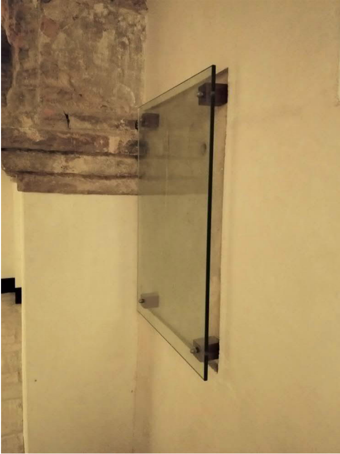
Fig. 1 Photograph of the graffiti protection system in the Torre del Trovador in the Aljafería Palace. Photo: Jorge Jiménez López
